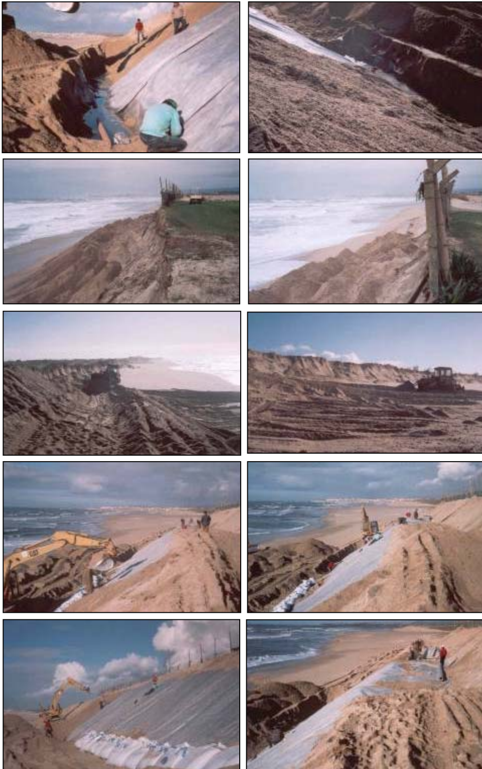
Fig. 19: Aspects of the execution of the technical solution using geotextile sand containers, December 2000.
